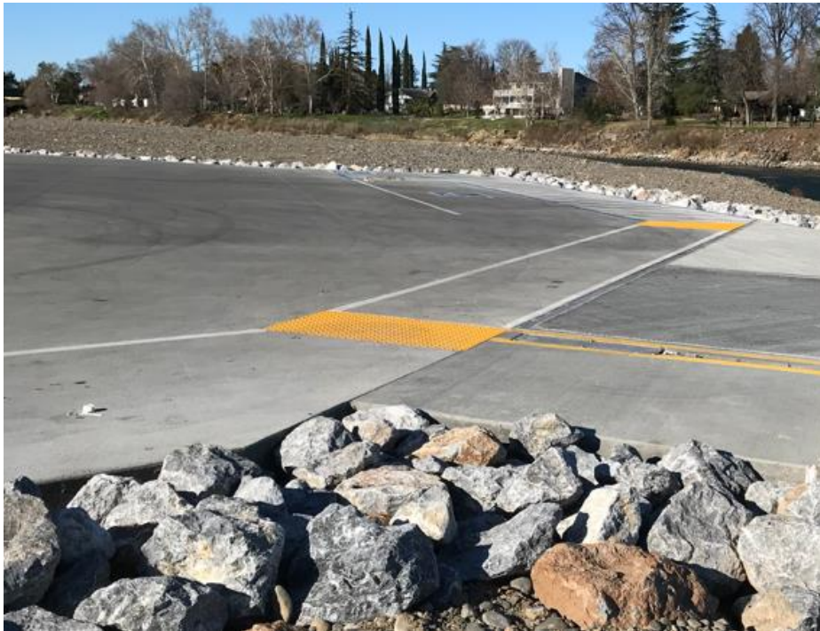
Accessible path of travel at the top of the boat launch ramp
